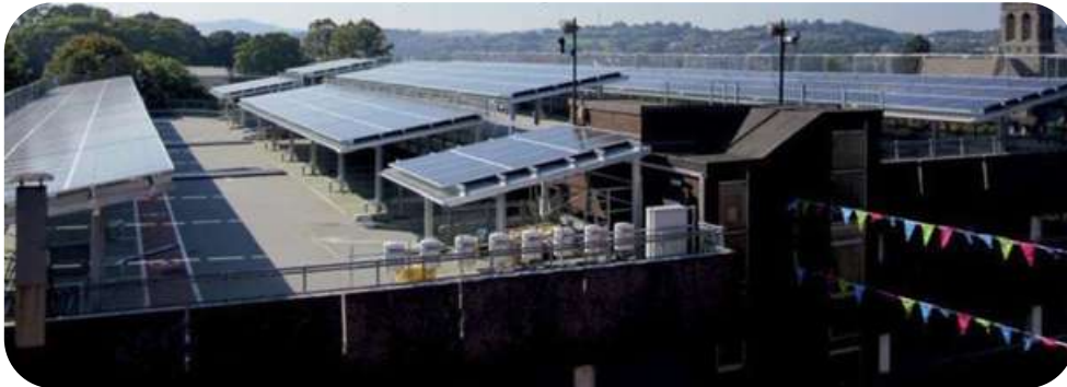
Photovoltaic array installed at Exeter's Mary Arches car park which has provided for a carbon positive building.
